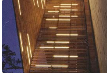
Strip lighting fixed to tunnel ceilings and walls
